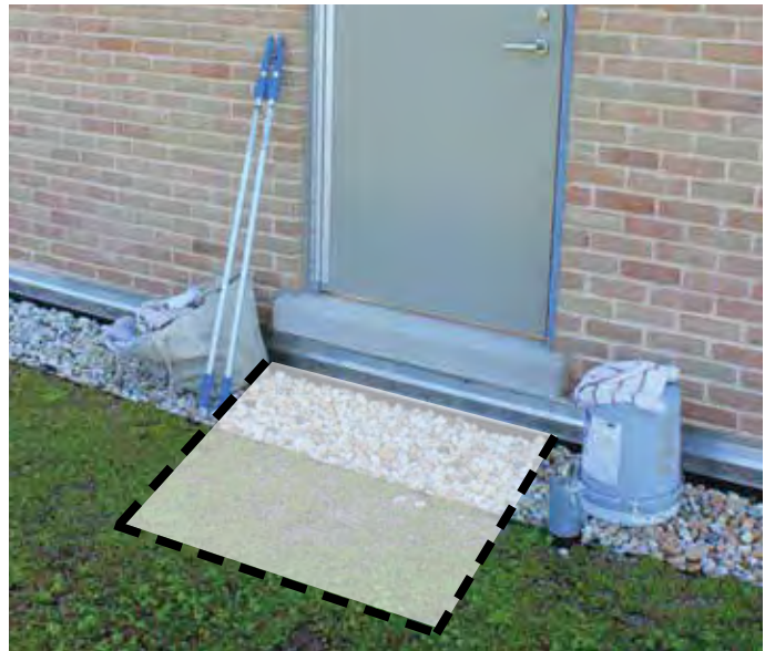
Landing pad needed at door
