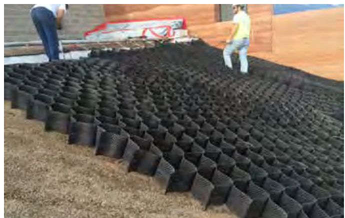
GardNet® used to stabilize LiteTop® media layer on sloped roof - Brinton Museum - Brinton, WY
