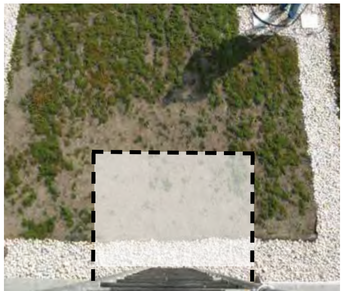
Landing pad needed at base of ladder
