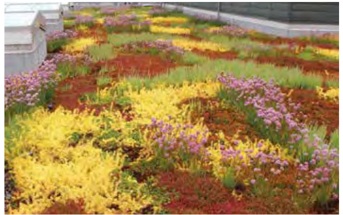
Tri-City Wastewater - Oregon City, OR
