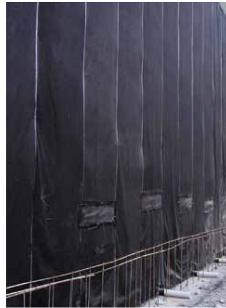
Underseal® Blindsid Membrane being installed over a timber lagging soil retention system utilizing Polyflow® 15 and Totalflow™.
