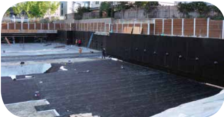
Underseal® waterproofing system utilized for entire foundation. Underslab (horizontal) installed with tie-in to Blindside (vertical).
